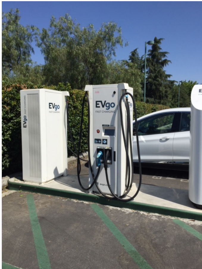
Installed ABB Unit
